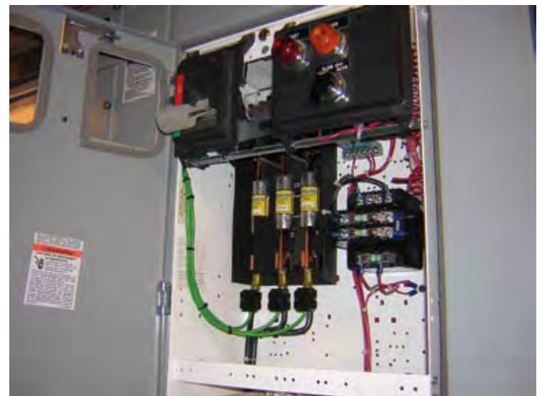
Figure 5 -Sensors installed on 200Amp disconnect.
