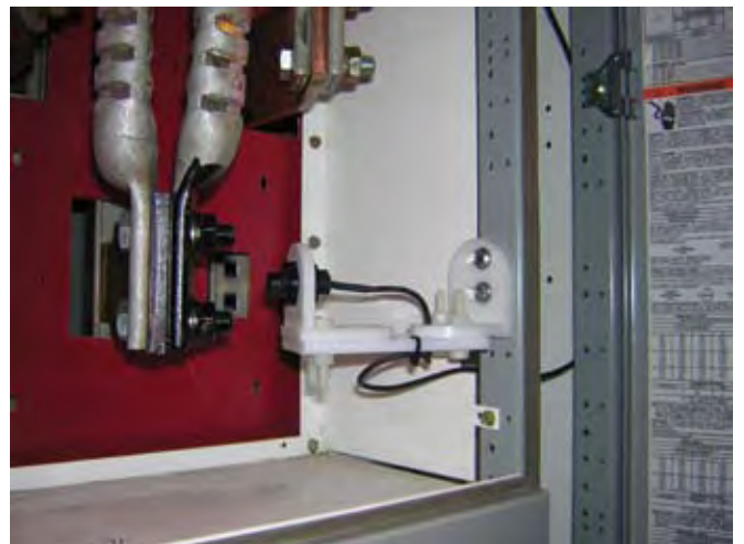
Figure 3 - Infrared sensor installed on 1 phase of a feeder to a panel.
